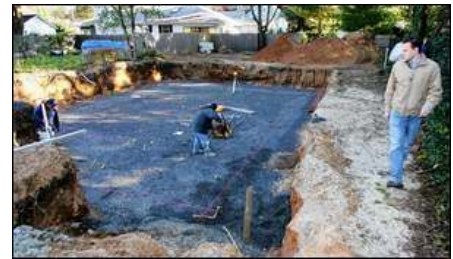
Andrew Calvo looks on as workers prepare a foundation for a modular home being built on Kemp Avenue in Fair Haven.
